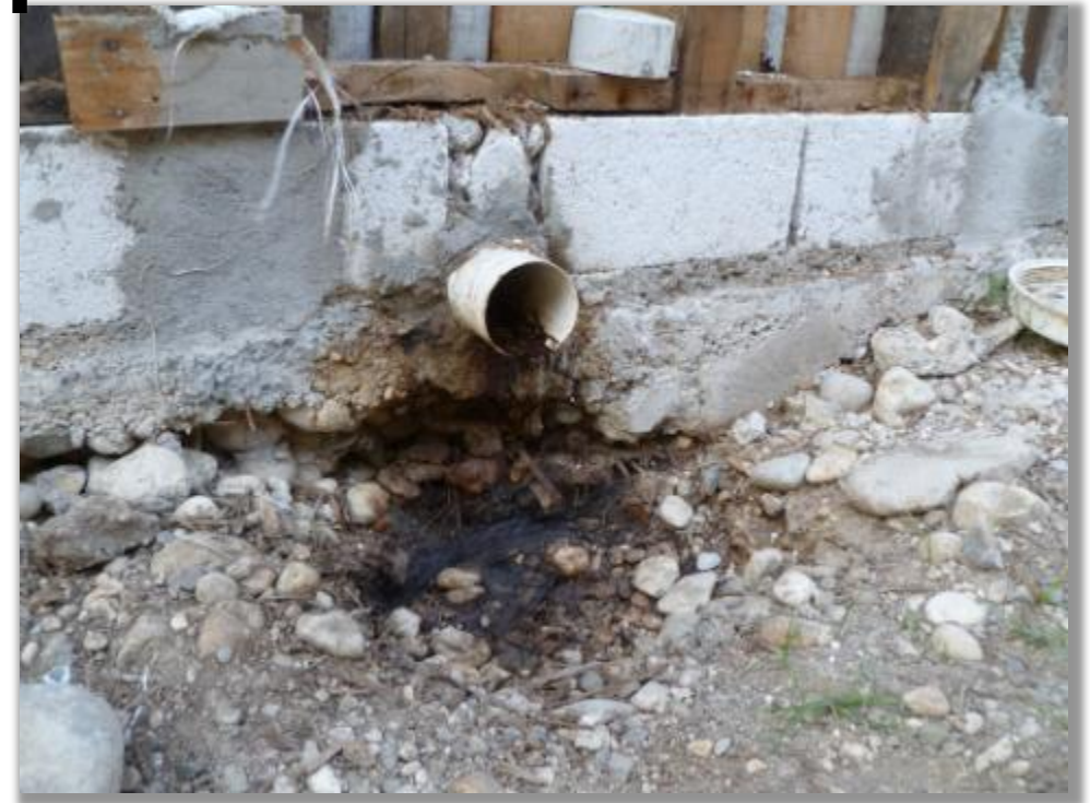
Photo K110: Jikaka leaking through space beneath leachate drain
